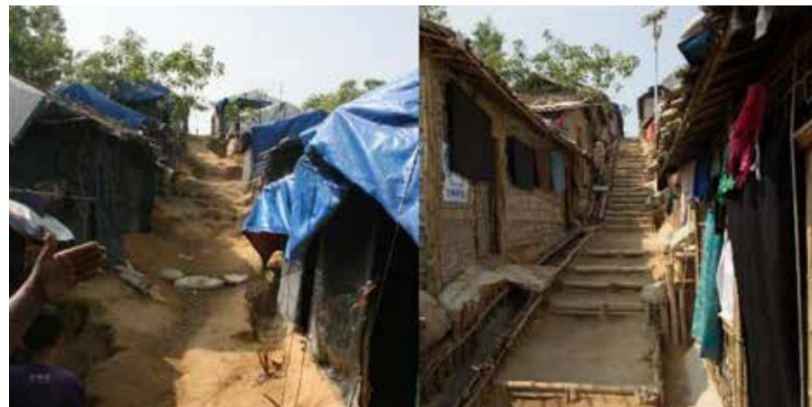
Before and after: Through a CRS cash-for-work activity, Rohingya refugees used locally available materials and techniques to build drainage structures and terraces to mitigate erosion and flooding in the refugee settlement. Photos by Christopher Reichert/CRS
