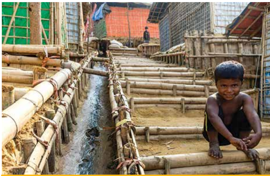
Through a CRS cash-for-work activity, Rohingya refugees used local materials to build structures such as drainage and terraces to mitigate erosion and flooding in the refugee settlement. Photo by Christopher Reichert/CRS
