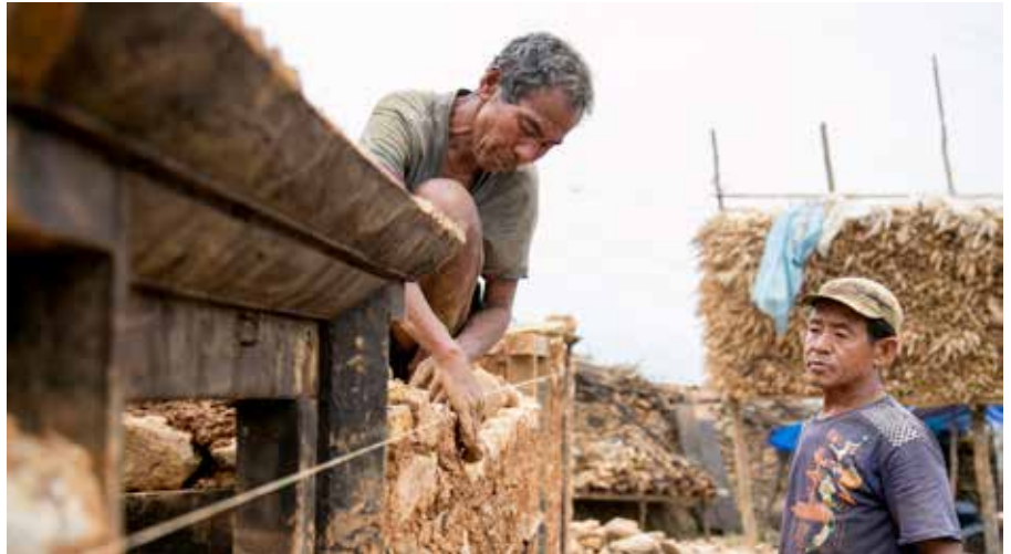
Dal Bahadur Rana Magar constructs an earthquake-resilient home in Gorkha after taking part in a CRS training. Photo by Jen Hardy/CRS
